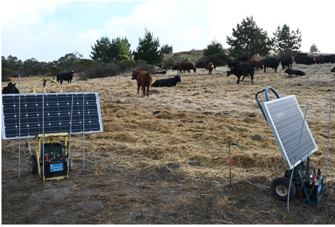
Energy for the hot wire
